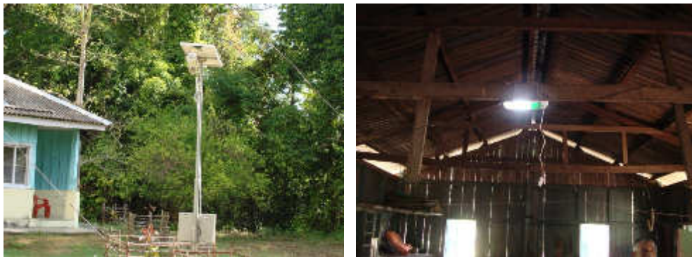
Fig-18 Solar electrification at Interview Island –Eastern Camp
